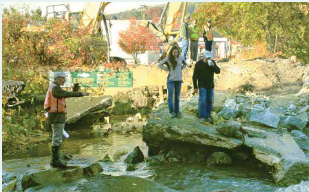
Director of Habitat Restoration Gwen MacDonald (center) and Green Projects Coordinator John Champion (right) monitored the removal of Pond Lily Dam, along with Michael Chelminski, Stantec Project Engineer (far left). These projects were led by Save the Sound, administered in partnership with the U.S. Fish and Wildlife Service, and funded in part by the Disaster Relief Appropriations Act of 2013 through the Department of the Interior, the Natural Resource Conservation Service, Trout Unlimited, the State of Connecticut and the National Fish and Wildlife Foundation.
